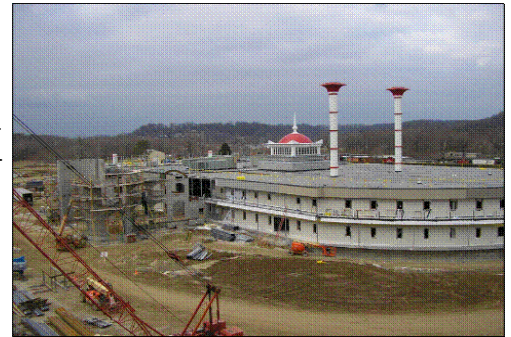
The top goes on the riverboat at the new French Lick Casino & Resort, scheduled to open in Orange County this December.
